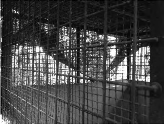
Figure 2: The roof and upper portions of the wall are made of 2 x 2 in galvanised iron mesh, overlaid with 0.5 x 0.5 in stainless steel mesh
